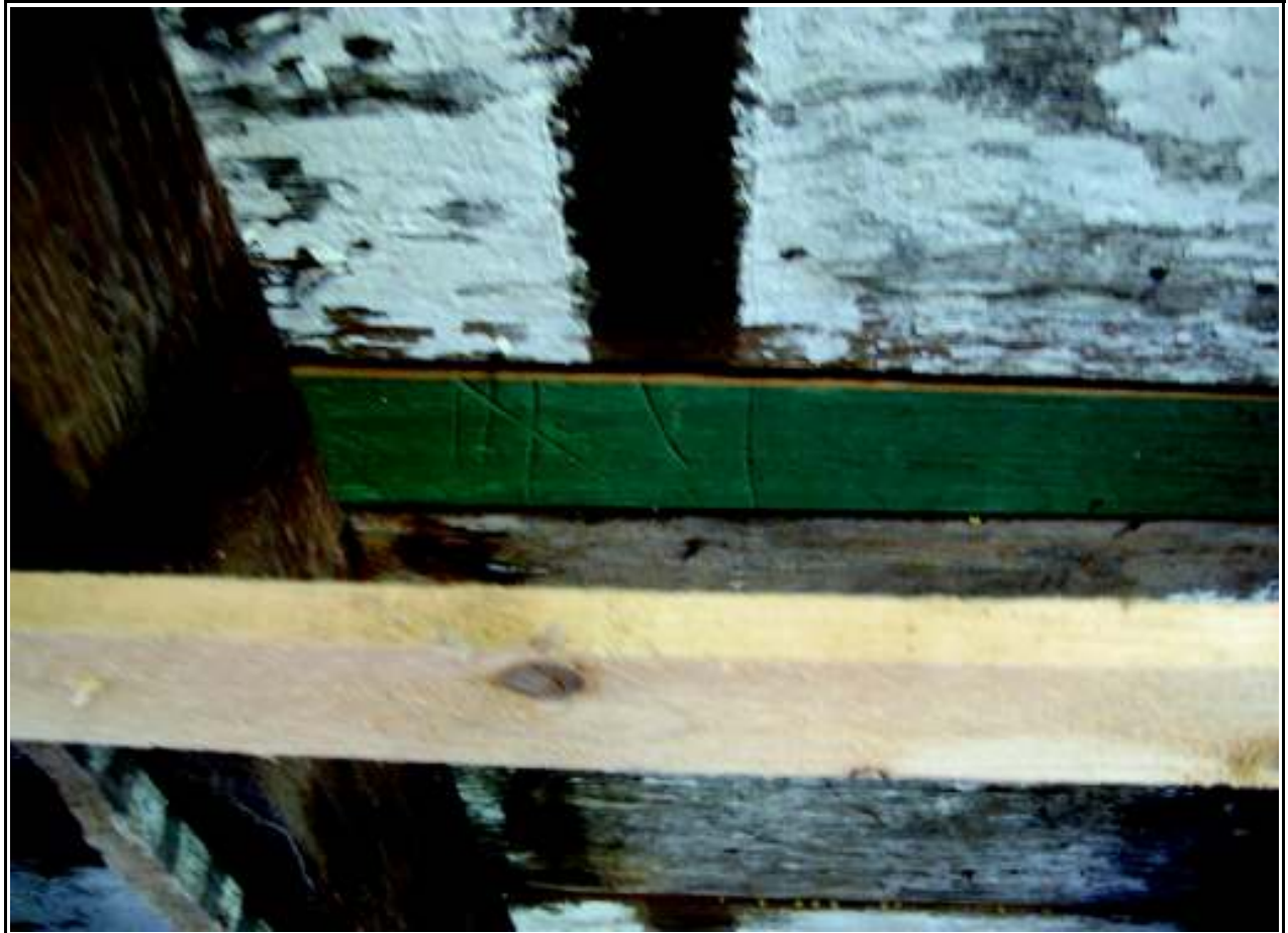
Figure 31. Whitewashed boards in attic
